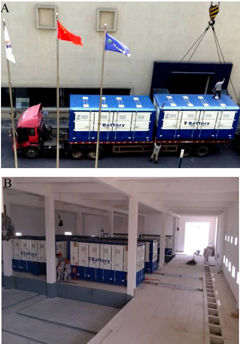
图 8 融科储能公司研制的 2 MW/4 MWh 集装箱式全钒液流电池储能系统吊装及现场安装照片 Fig. 8 Photographs showing the RKP's 2 MW/4 MWh containerized VFB system developed by PKP (A) and the field installation of the system (B)
